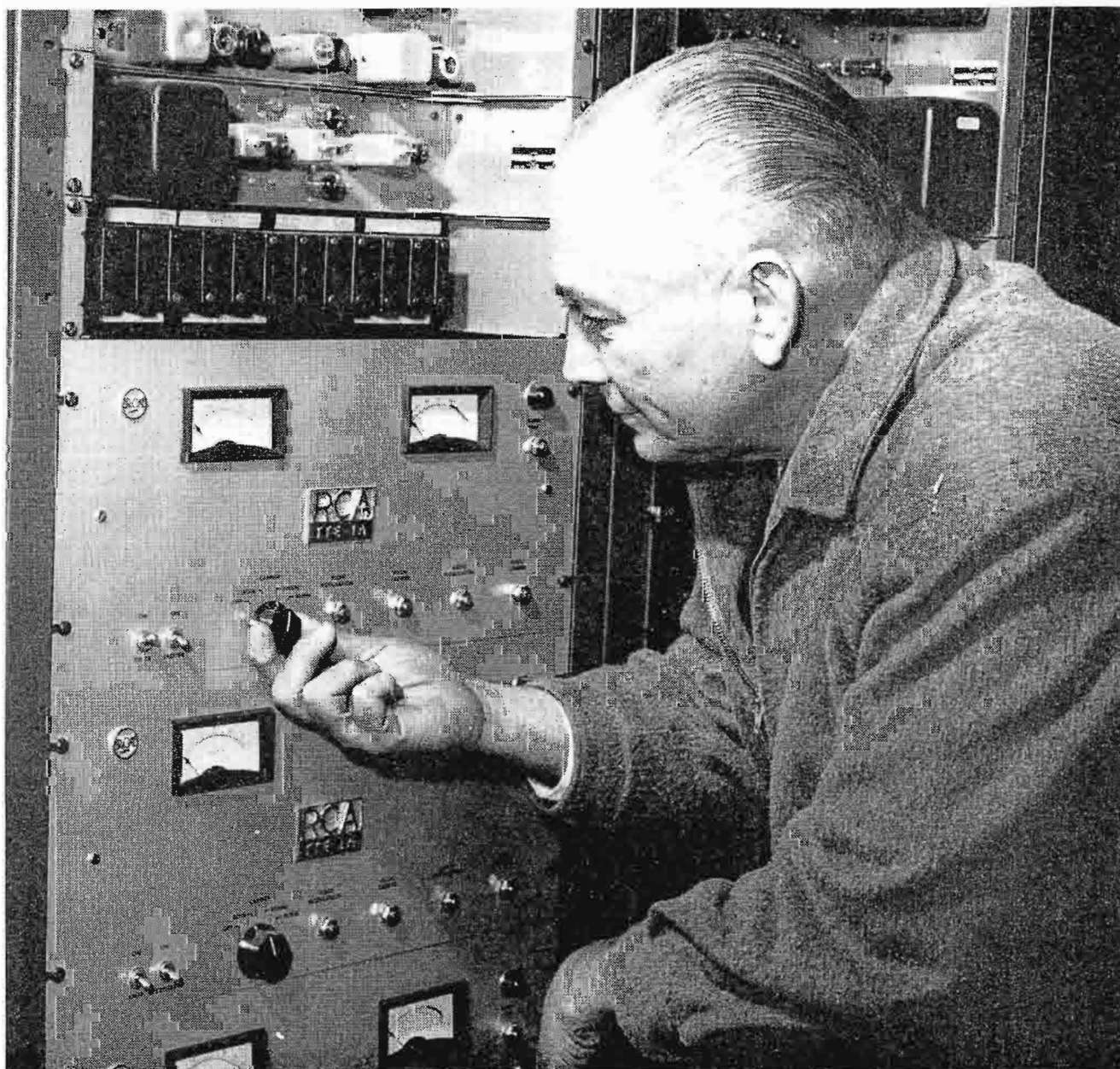
FIG. 3. A portion of the RCA 2500 MHz transmitter equipment installed at the Communications Center at St. Joseph's Seminary in Yonkers, New York a part of the Archdiocese of New York ITV System.
